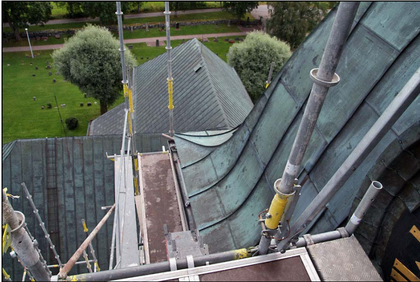
Nedre takfallet innan restaurering.
